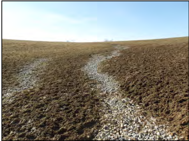
Photo 6: View of the swale filled with gravel on the north end of the site, looking southwest.
